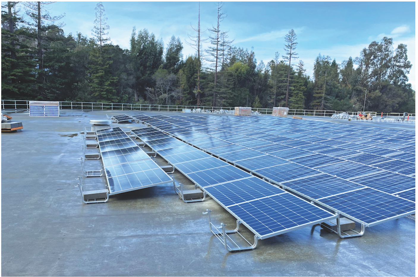
SUN STYLE – The Vickery Station in Saratoga can generate 510 megawatt-hours of electricity a year. (Courtesy of SJ Water)
