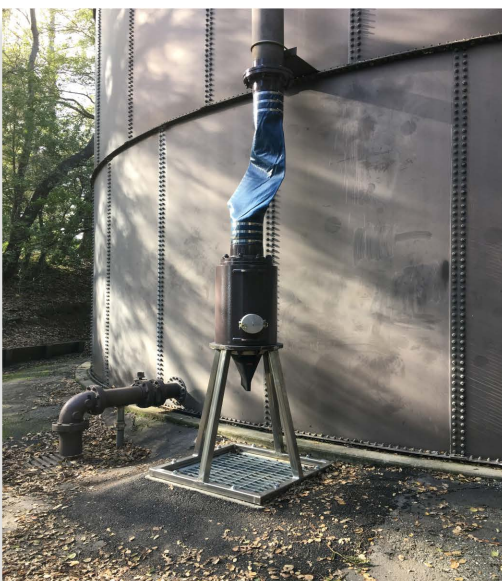
A new Dechlorinating Overflow Security Assembly (DOSA) installed at one of SJWC's water tanks
