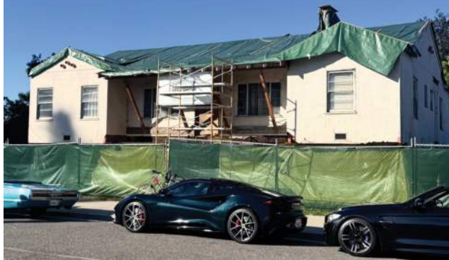
The Sakaue Family Farmhouse, photographed Wednesday, was saved from demolition and moved to History Park in San Jose. A fundraising effort is underway to restore it. SAL PIZARRO — STAFF
